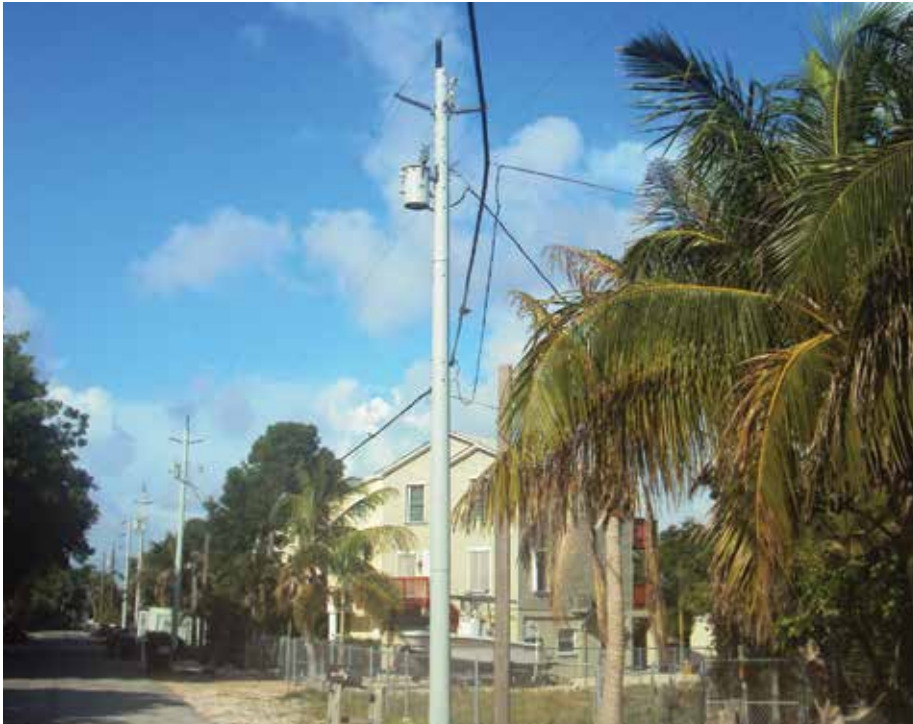
▶ Corrosive Environments & Coastal Areas
